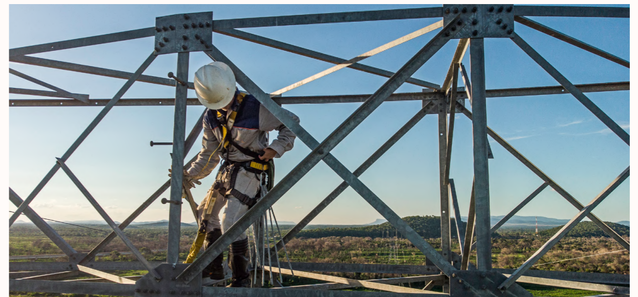
Energy work in PATE
