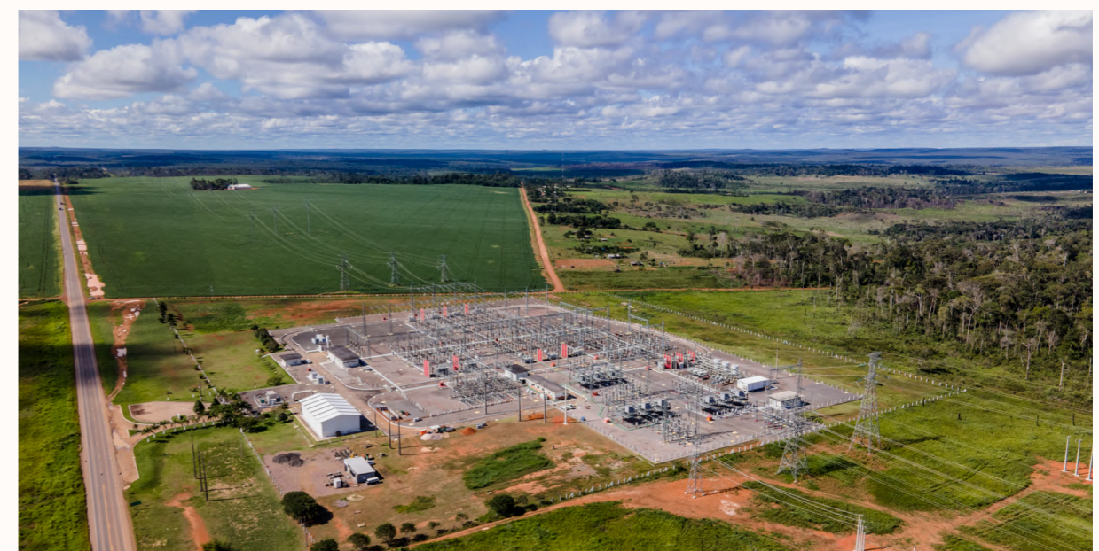
Vilhena substation, JTE
