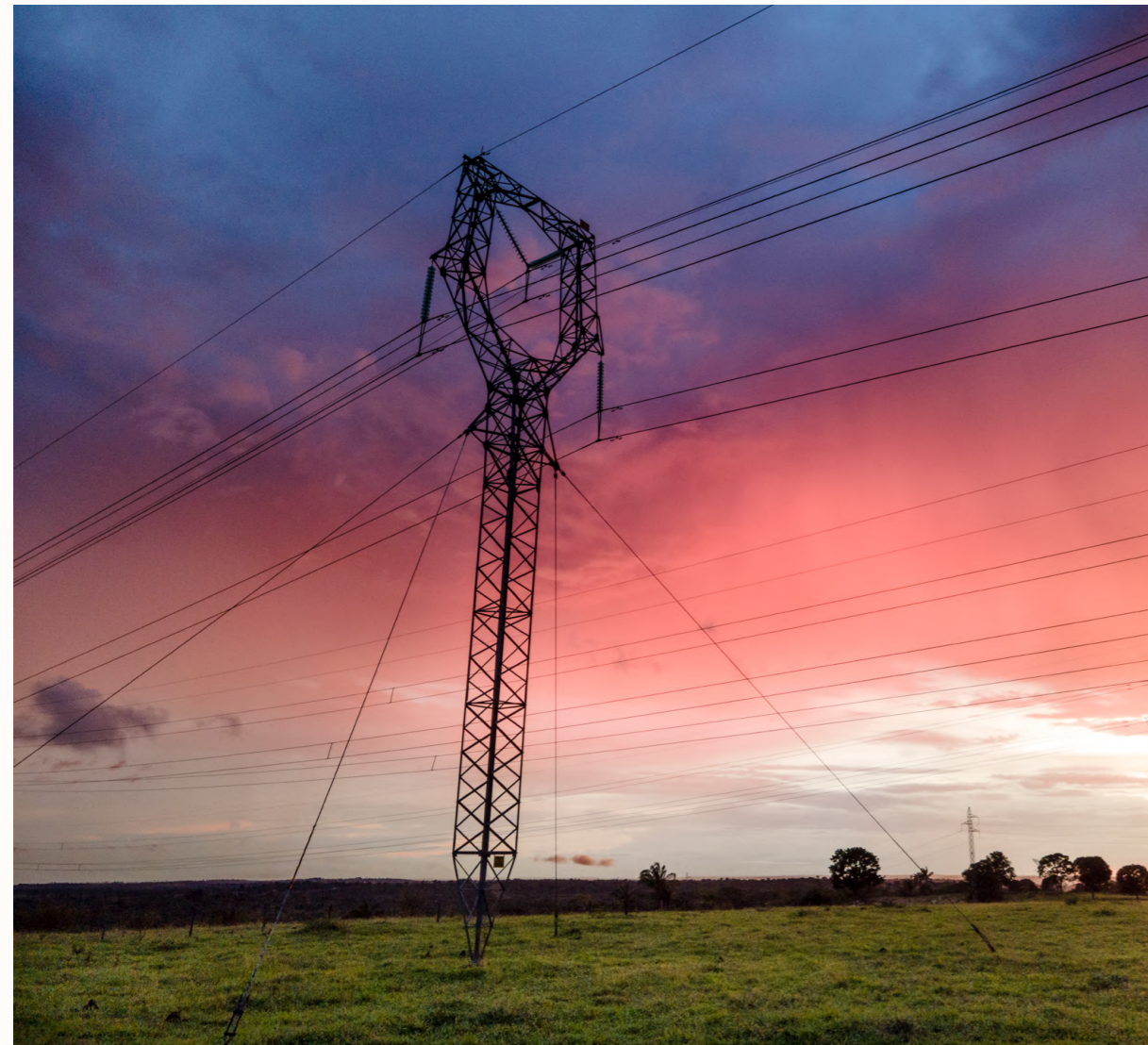
Jauru transmission line
