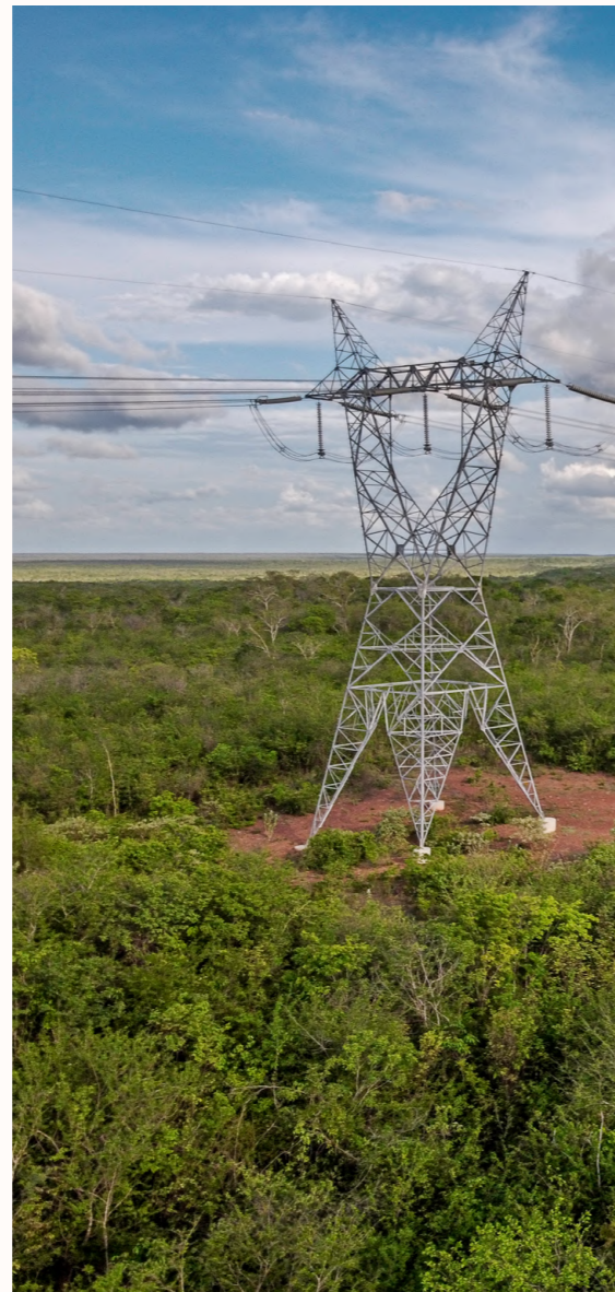
SITE transmission line
