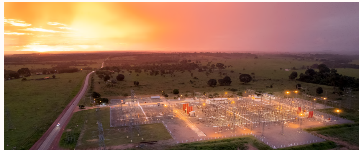
Pimenta Bueno substation, JTE
